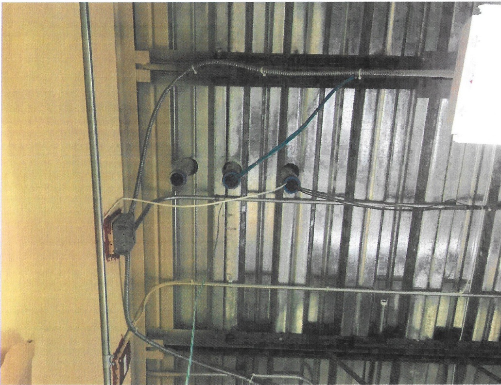
Image 2: There are various conduit routes through the floor and ceiling from the IDF to other parts of the school that could possibly be used to route the GPS antenna cable.
